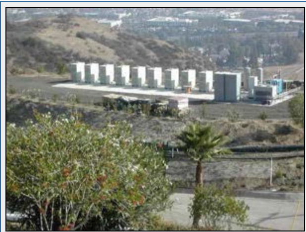
300 kW microturbine facility at Calabasas landfill
