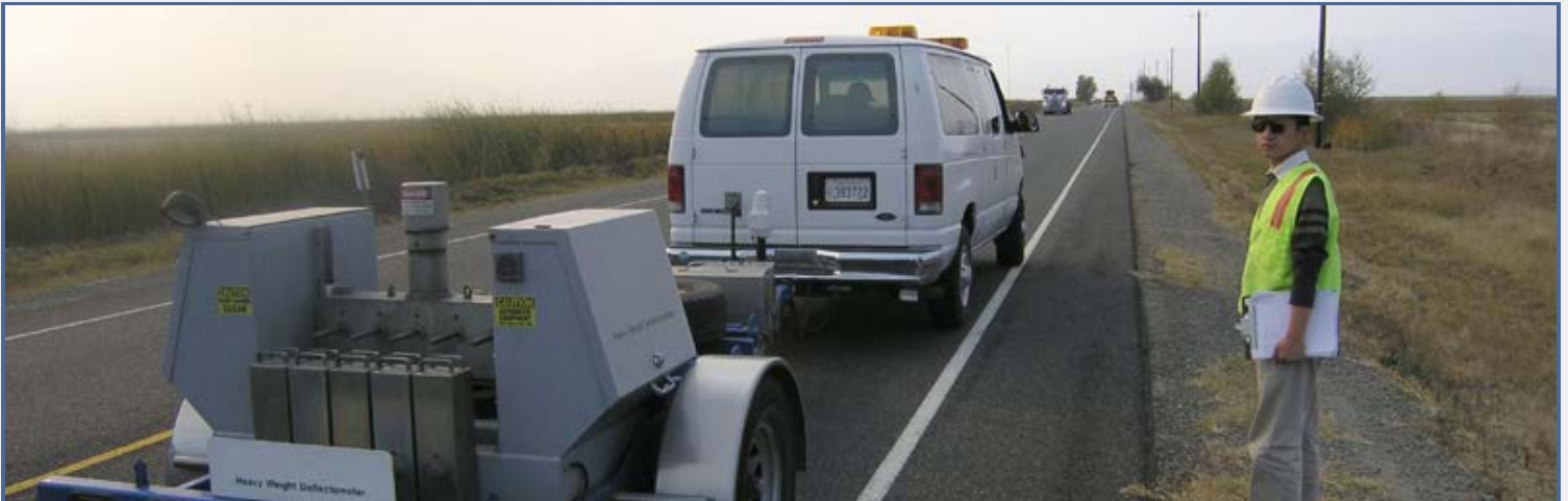
Pengcheng Fu at work on SR33 in Colusa County, the first Caltrans project using FDR-foamed asphalt
