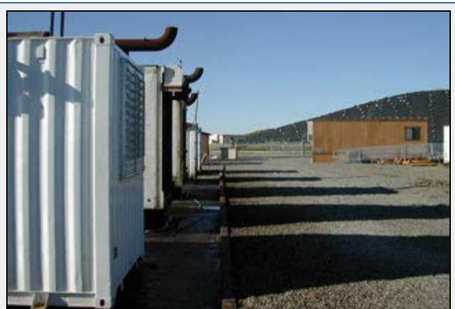
Landfill gas-to-electricity bioreactor
